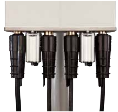
Multiple 3M™ Slim Lock Closures installed on a Multiple In Multiple Out (MIMO) antenna.
